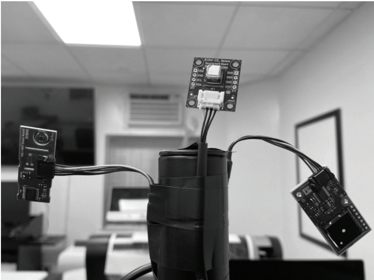
Air quality sensors from Loisaída's sensor lab. Volatile organic compounds (VOC)/Relative humidity and temperature sensor (left), CO 2 sensor (center), Formaldehyde sensor (right). (Alex-Nicole Edwards)
